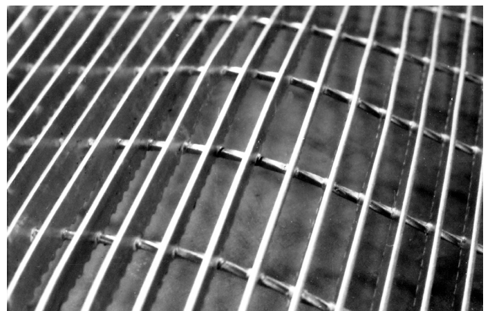
Fig. 15 - Closeup of Impact Damage to Steel Grating
